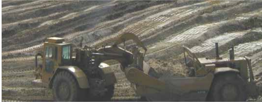
Rates of erosion increase dramatically during construction.
