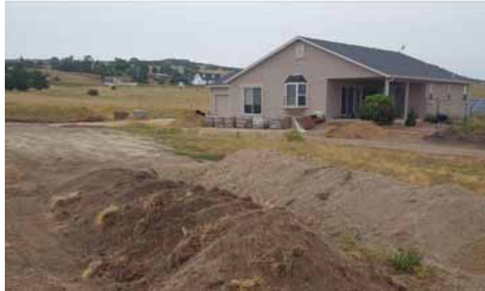
The Low Impact GESC Permit issued for a rural residential property to construct a small berm (grading in progress).
